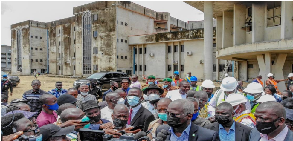
Hon. Minister of Works and Housing, Mr Babatunde Fashola, SAN (middle) speaking with journalists shortly after inspecting the ongoing construction of the Federal Secretariat Complex, Yenagoa in Bayelsa State on Tuesday, 28th September 2021.
