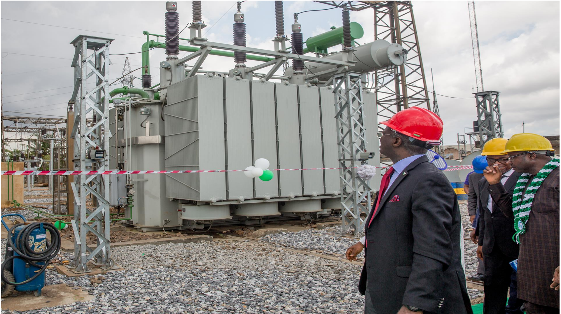
Hon Minister of Power, Works & Housing Mr Babatunde Fashola, SAN (left) and Managing Director/CEO, Transmission Company of Nigeria (TCN), Mr Usman Gur Mohammed (middle) inspecting one of the transformers during the commissioning of the 2 x 100MVA, 132 /33KV Power Transformers at the Ejigbo Transmission Substation, Ejigbo L.C.D.A (Oshodi/Isolo LGA) Lagos State on Thursday 18, October 2018.
