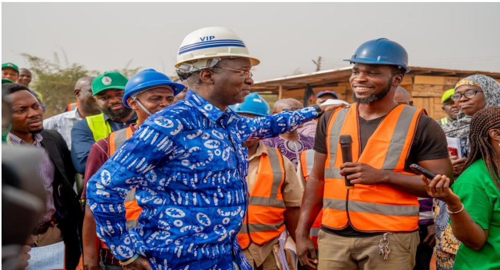
Hon. Minister of Works & Housing, Mr Babatunde Fashola, SAN (left) interacting with the Foreman on Site, Mr Obinna Onyeka (right) during the inspection of the progress of work at the National Housing Programme Site in Delta State on Tuesday, 11 th February 2020.
