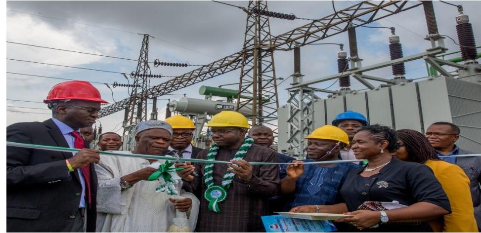
Hon Minister of Power, Works & Housing Mr Babatunde Fashola, SAN(middle) and others during the commissioning of the 2 x 100MVA, 132 / 33KV Power Transformers at the Ejigbo Transmission Substation, Ejigbo L.C.D.A (Oshodi/Isolo LGA) Lagos State on Thursday 18, October 2018.
